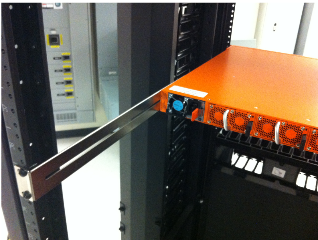
Figure 6 Rear View of the Mounted Node and Rails on the Four-Post Rack
